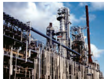
蒸留塔 Fractionating column
